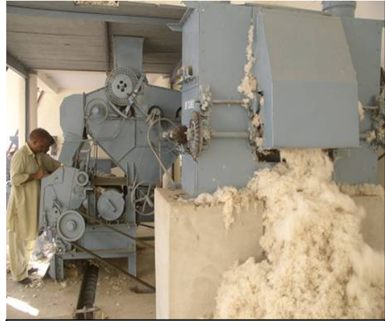
CIPHET Cotton Ginning Plant in operation
