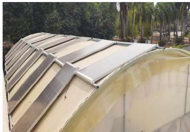
Fig. 47. Installation of Solar Panel on Roof of Fan Pad Cooling Poly House
