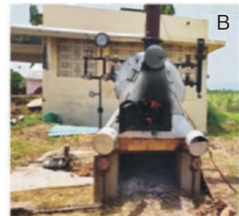
Furnace & Steam boiler
