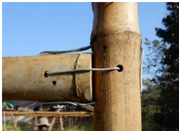
Fig. 42(a). Side joints between bottom chord and side column
